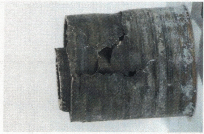
Figure 23 – Leak, Coil Sample 1
